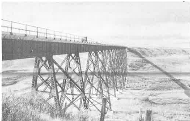
One of four large trestles on the Central Montana RR (Indian Creek).
