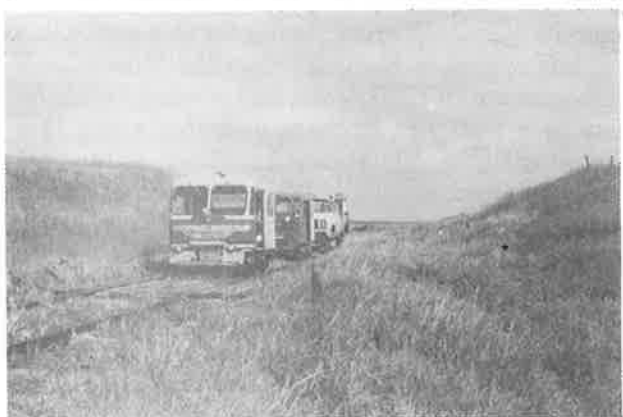
The work crew at the newly constructed motorcar turnaround, approximately three miles west of Oakaton, South Dakota.
